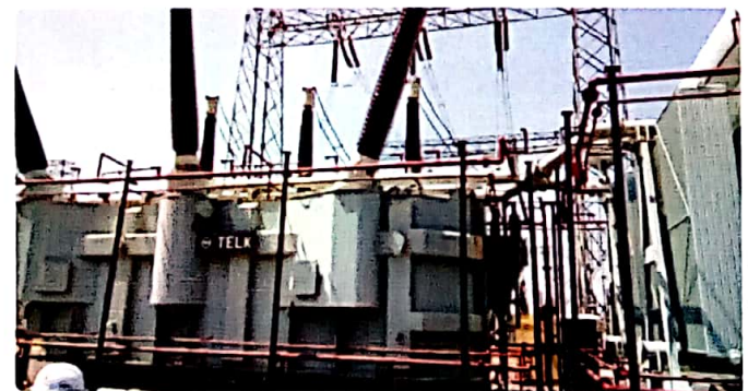
Transformer at the Substation
